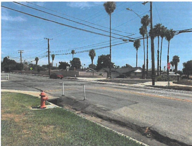
Elevated sidewalk with large gutter entry way along the City's cooperated boundary presents an opportunity to collaborate with surrounding Agencies to improve roadways. (Pacific Street near Highland Pacific Elementary School).
