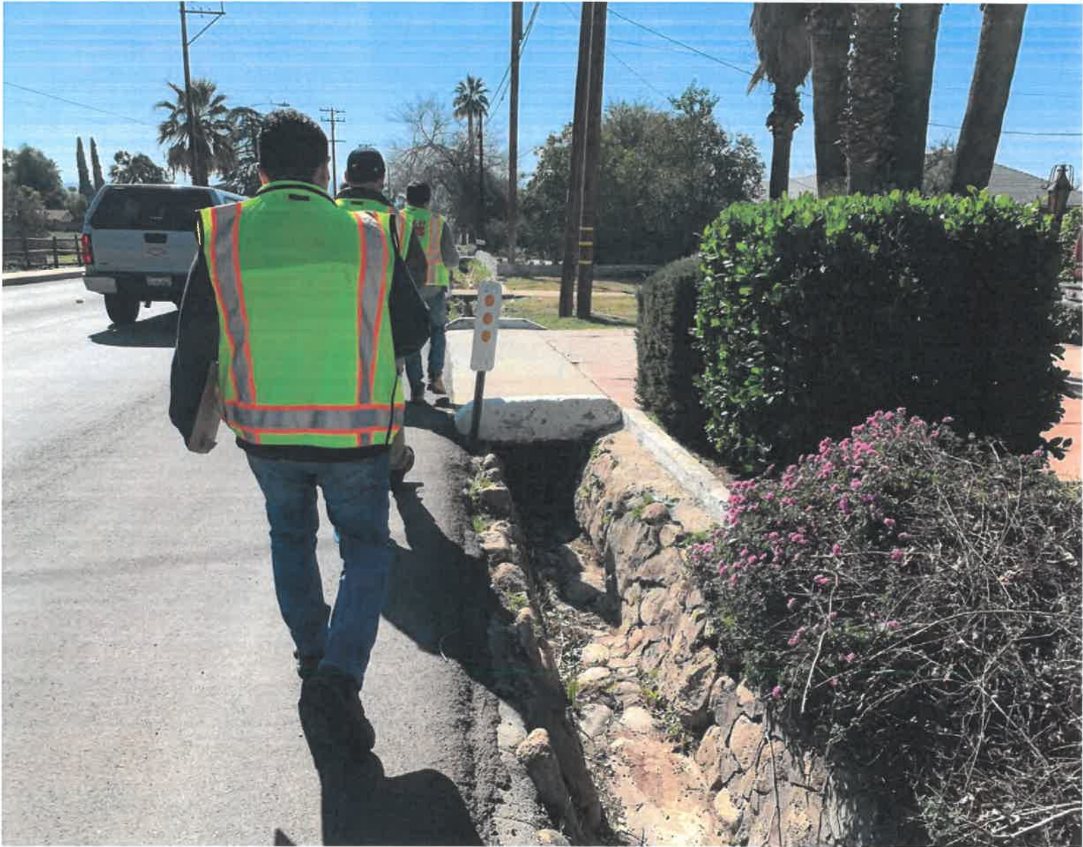
Much of the western side of Palm Avenue between Main and Messina Streets lack sidewalks.
