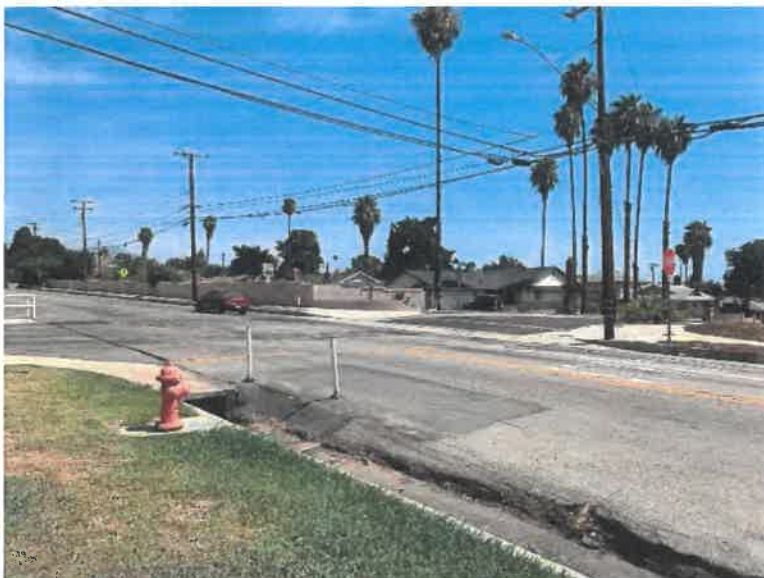
Elevated sidewalk with large gutter entry way presents hazardous conditions (Pacific Street near Highland Pacific Elementary School).
