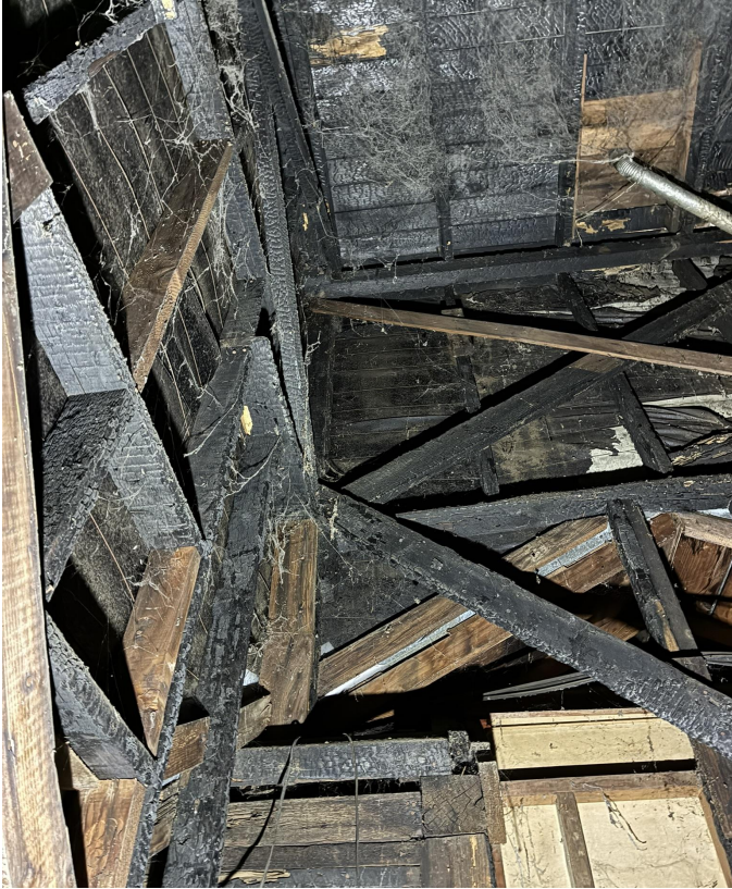
FIGURE 13. FIRE DAMAGE AT EAST BELL TOWER WALL
