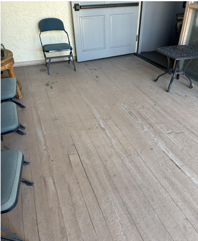
FIGURE 4. FAILED WATERPROOFING OVER EXISTING WOOD DECKING
