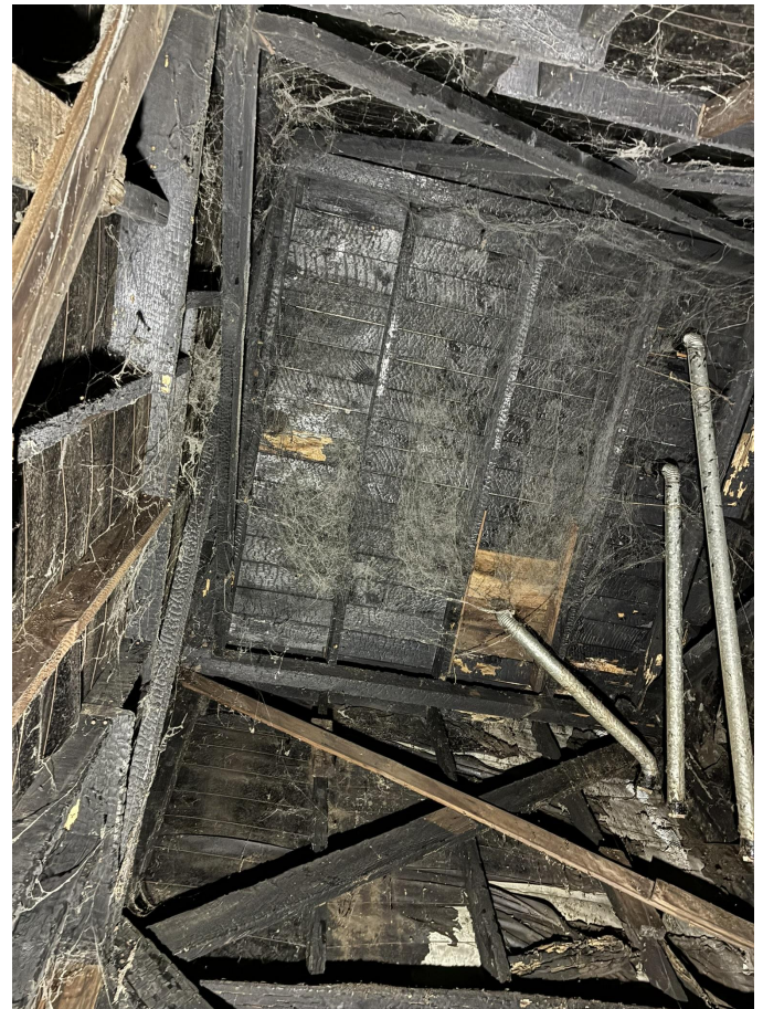
FIGURE 12. FIRE DAMAGE AT TOP OF BELL TOWER
