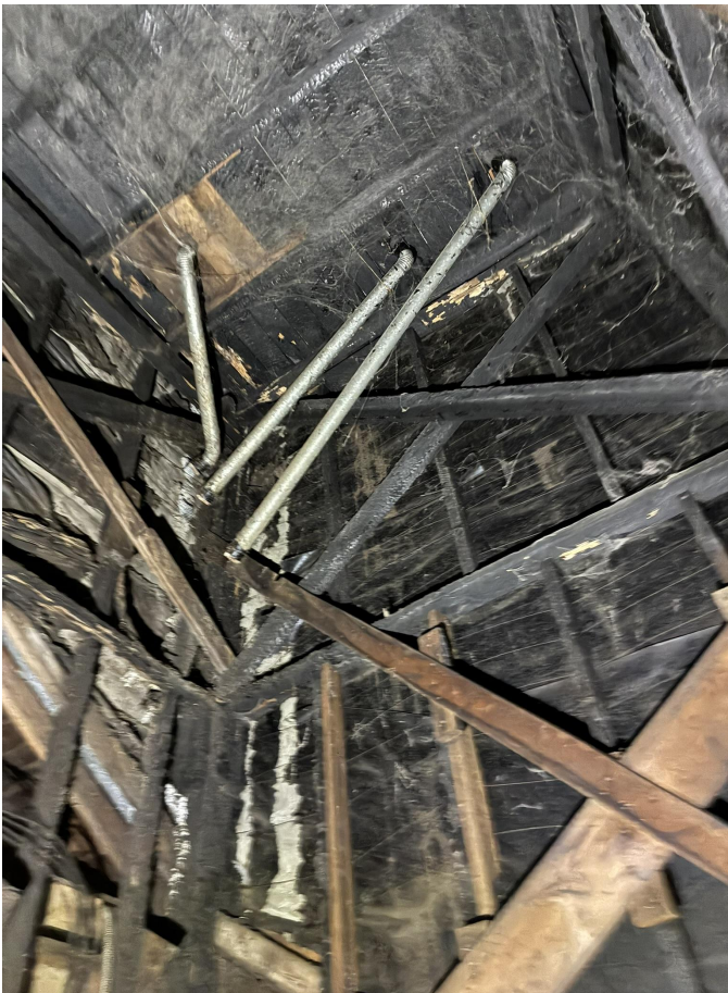
FIGURE 11. FIRE DAMAGE AT SOUTH BELL TOWER WALL
