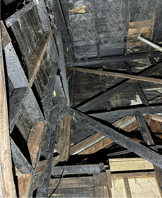
FIGURE 13. FIRE DAMAGE AT EAST BELL TOWER WALL
