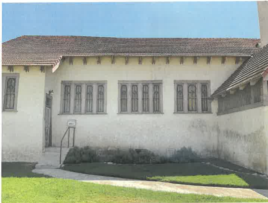
FIGURE 1. WATER STAINING ON STUCCO, AND PLANTER NEARBY FOUNDATION
