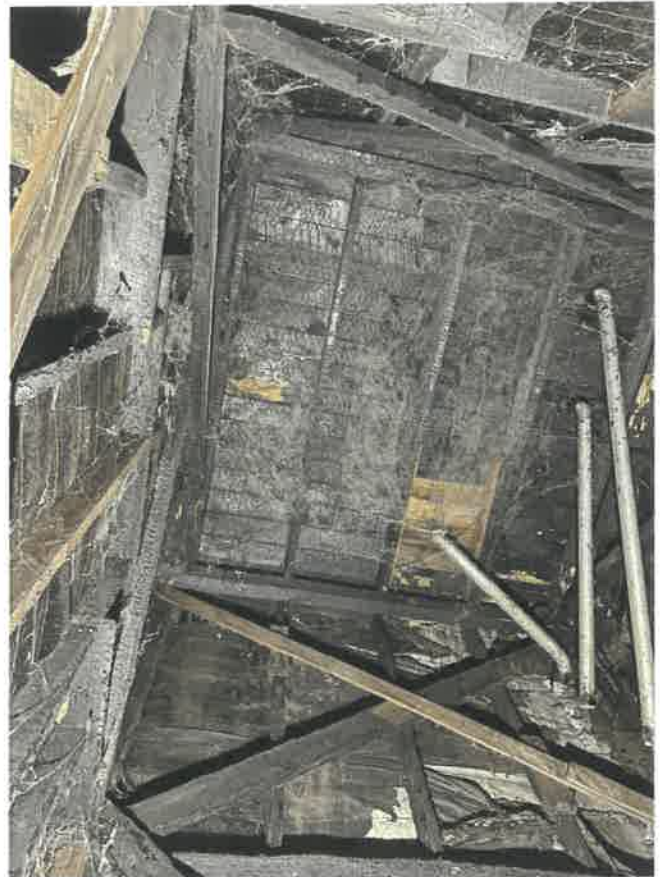
FIGURE 12. FIRE DAMAGE AT TOP OF BELL TOWER
