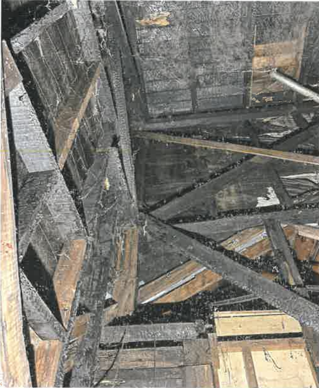
FIGURE 13. FIRE DAMAGE AT EAST BELL TOWER WALL
