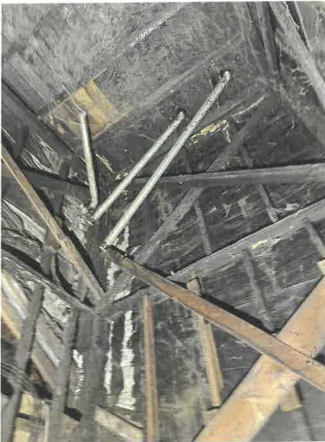
FIGURE 11. FIRE DAMAGE AT SOUTH BELL TOWER WALL
