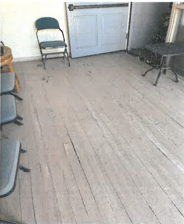
FIGURE 4. FAILED WATERPROOFING OVER EXISTING WOOD DECKING
