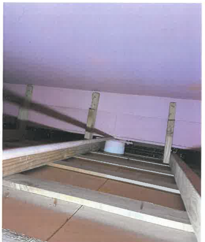
FIGURE 10. BEAM BRACING ROD INTERSECTING COLUMN SUPPORT
