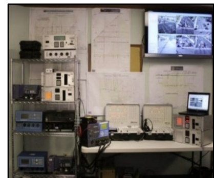
Traffic Signal Operations Lab
